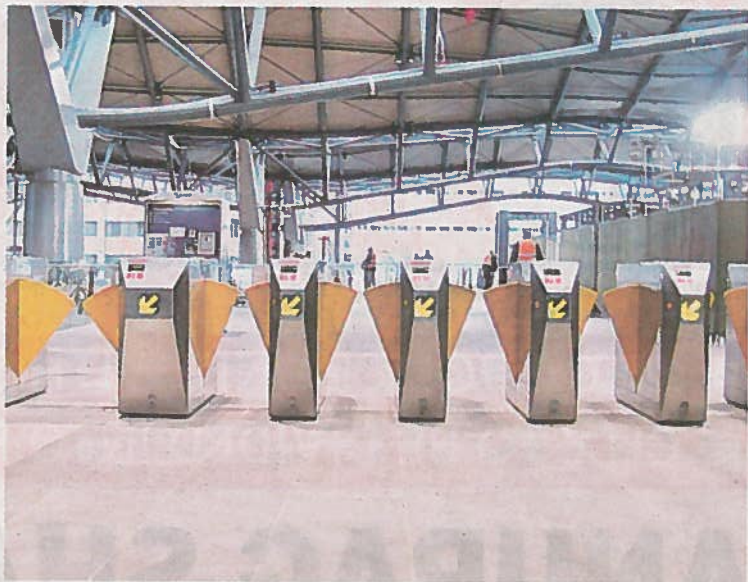
An Automatic Fare Collection barrier gate
