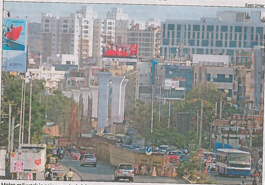
Metro rail work is going on at a brisk pace at Hi-Tec City
