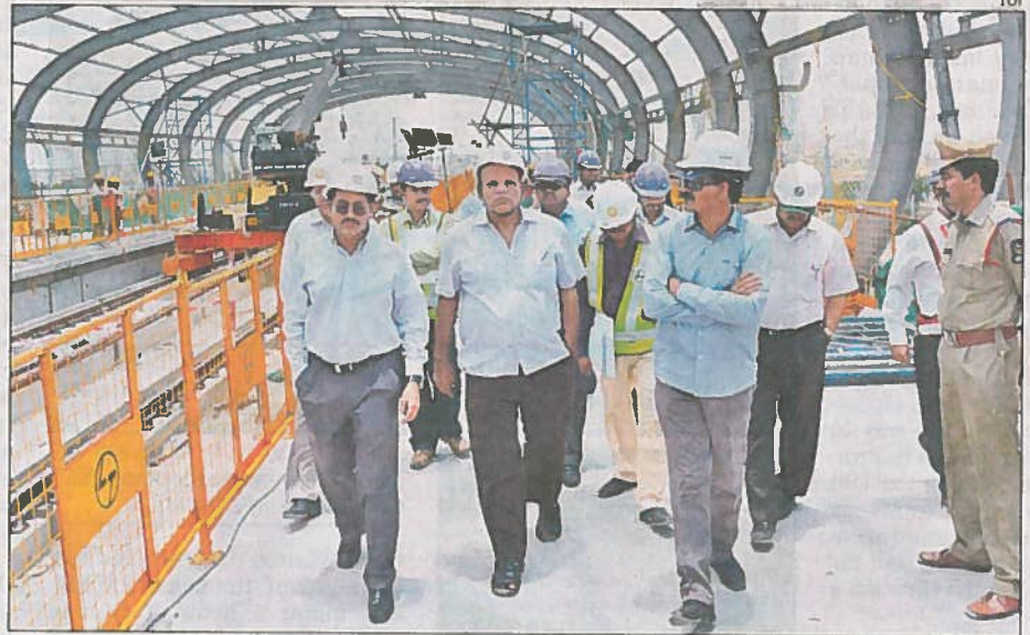
GHMC commissioner Somesh Kumar inspects under-construction metro rail station at Nagole on Tuesday. Metro rail MD NVS Reddy is also seen
