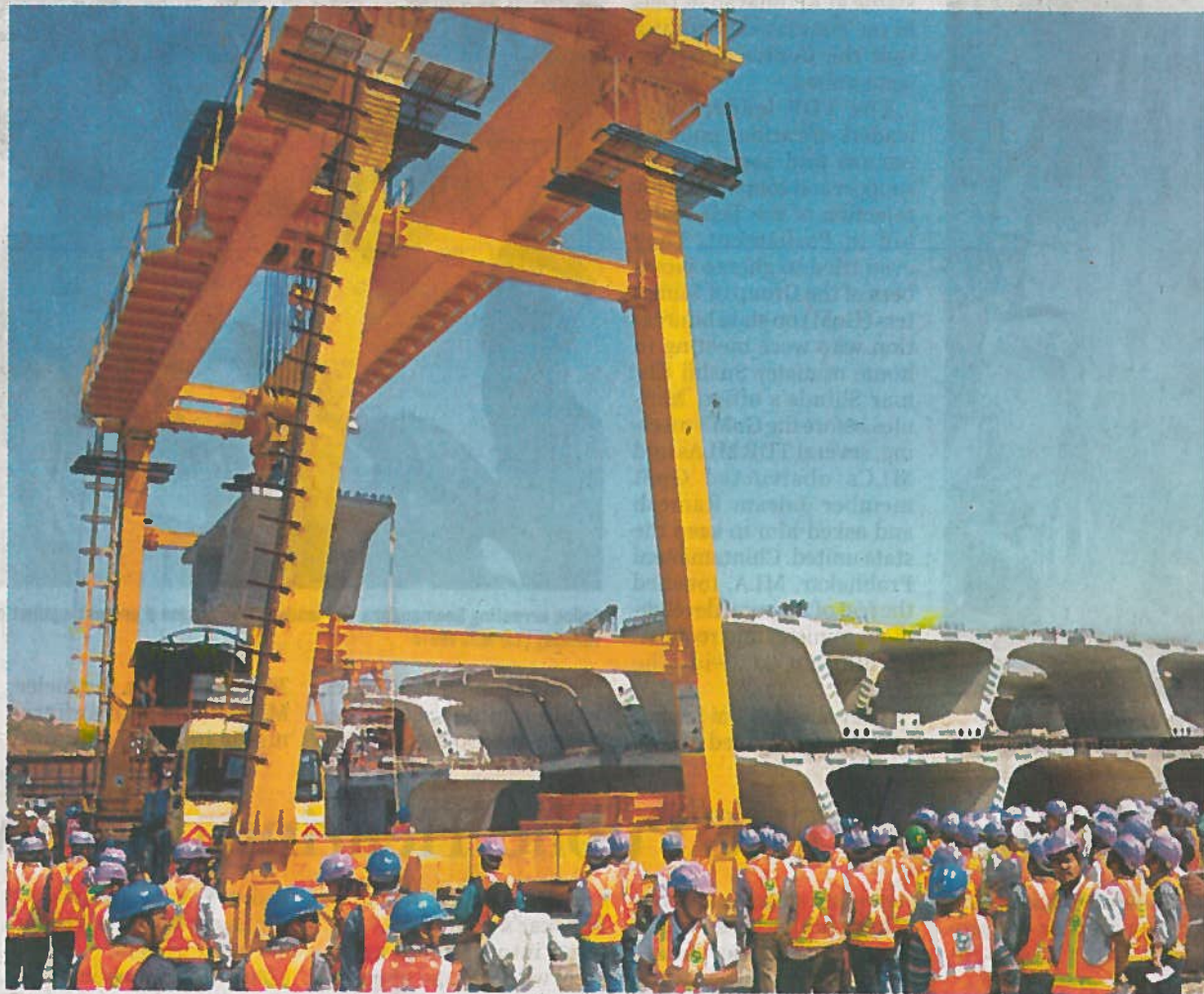
Viaduct segments for Hyderabad Metro Rail project being manufactured at Quthbullapur casting yard in Hyderabad on Tuesday | RVK RAO
