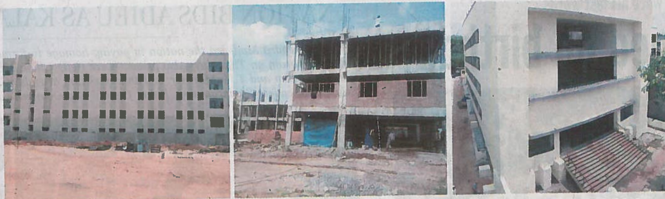
(From left to right) A new building built to house a school at Kukatpally. Construction of police barracks behind Shahinayatgunj police station complex under way. The commercial complex ready for opening at Putlibowli.
