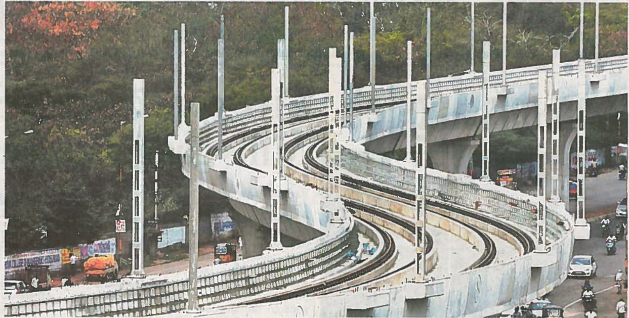
The Metro Rail viaduct will run parallel to flyovers, fly over several others, including railway overbridges.
