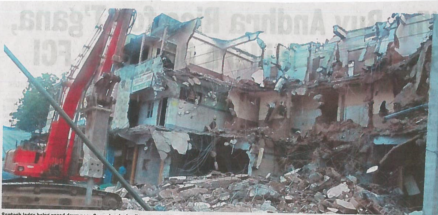
Santosh lodge being razed down near Secunderabad railway station on Tuesday | EXPRESS PHOTO
