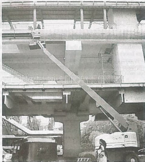
Metro rail station work at Habsiguda is progressing at a rapid pace in Hyderabad on Saturday | A RADHAKRISHNA
